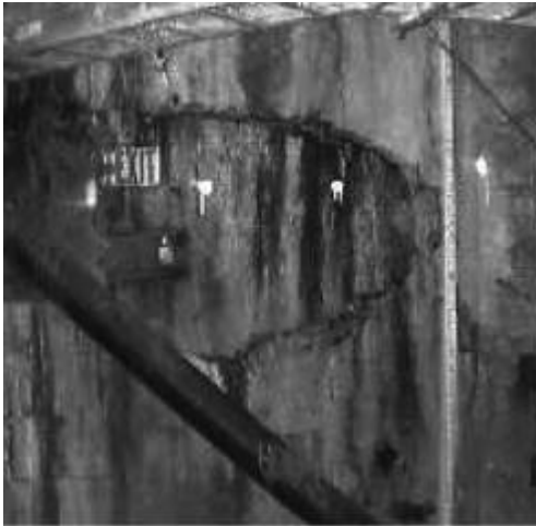
Figure 2: Cracking and staining observed on north wall of AST
